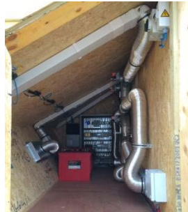
Control System – regulates temperature and selects heating method
